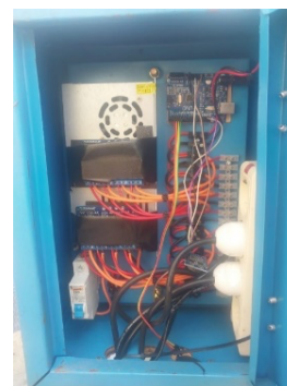
Fig 4. Control system electrical panel
